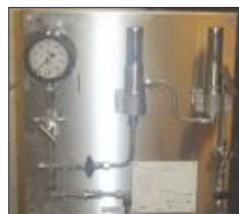
Valve Seat Leak Indicator Panel
